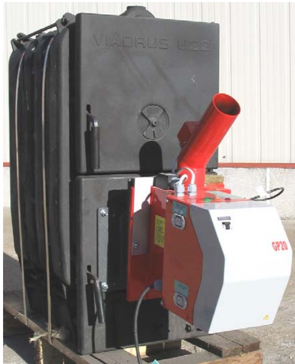
Figure 1.4.7. Automatic pellet burner of series “GP” is installed on transition flanged, attached at the lower door of the hot water boiler “VIADRUS U22” ( the picture shows a boiler without any covering plates );
